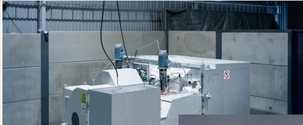
TES.POD units are clustered together to provide facilities with the required capacity.
